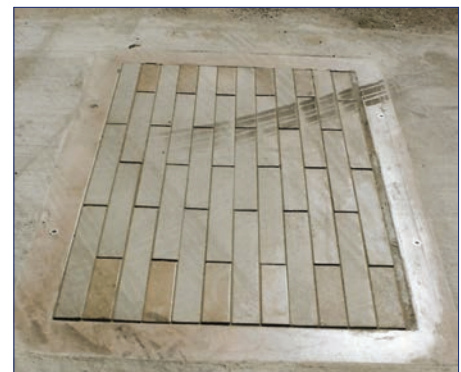
Skid marks on top of pavers show evidence of deliberate attempts to disturb installation. The mortar-set Narrow Modular Pavers held fast and were not dislodged by vehicular traffic.
