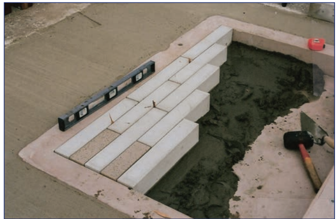
The precast concrete 27/8" x 177/8" x 4" Narrow Modular Pavers were set in a 1" mortar bed. Pavers were cut to fit to provide a staggered bond joint pattern.
